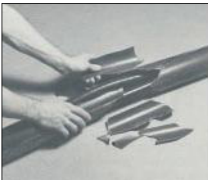
Remove damaged or faulty ducting
